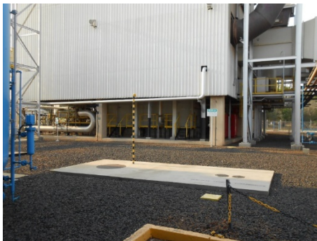
Figura 6 - Sump tank na ECOMP
